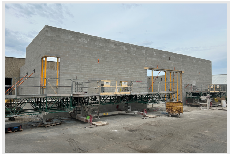
Findorff masons have completed the masonry building structure at the Skills Lab Addition. Structural steel will follow in the coming days.
